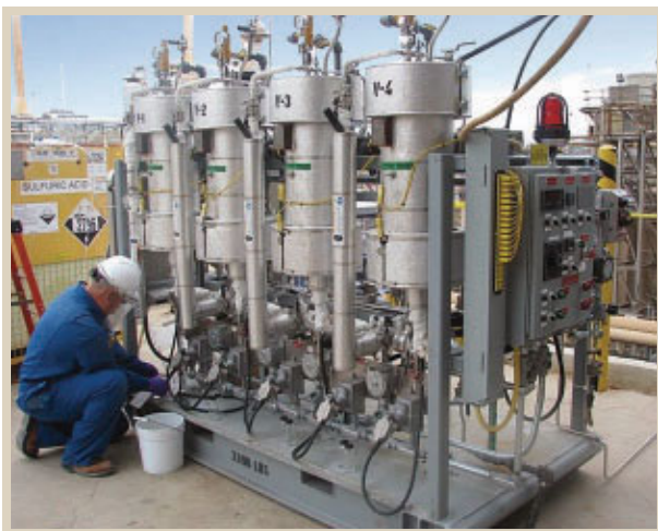
Mike Corbett, a technician from the Bartlesville Technology Center, collects a water sample from the selenium removal equipment. We are testing this technology in our Rodeo refinery.
