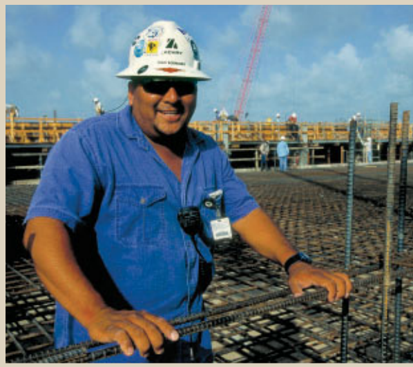
Rigo Rodriguez pauses from construction of the Freeport LNG terminal, the country's first new LNG terminal in more than 30 years.
