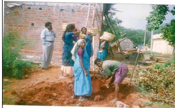
The widows are working as labours in the construction spot under the hot sun.
