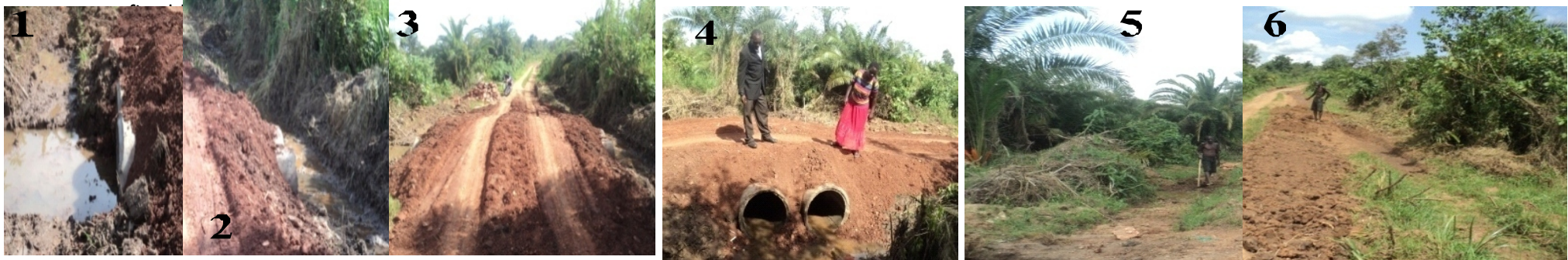
1,2,3, shows drainage and village road renovation Campaign by TWADDI, 4 members watching work done on the road which was impassable, 5 & 6 campaign to clear village roads
